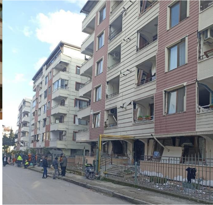
After the earthquake on 6 February
